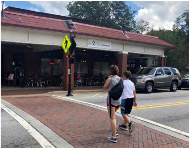
Rectangular Rapid Flashing Beacon (RRFB)
