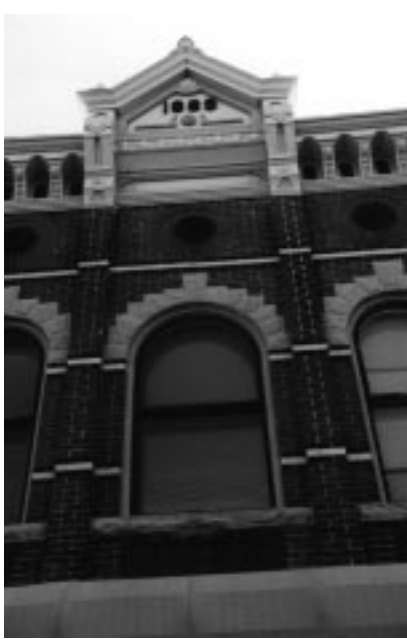
This 1889 building features a stone-arched window, decorative brick banding, and an elaborate cornice.
