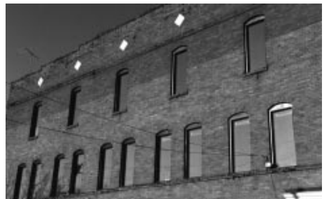
The original windows in this building have been replaced with fixed tinted glass; this change alters the historic appearance of the building.
