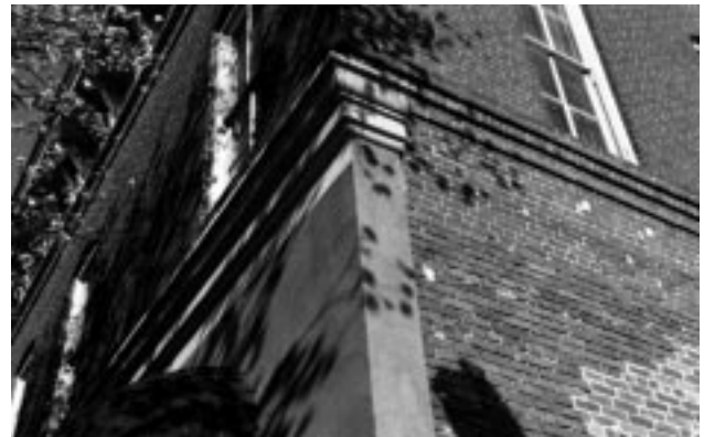
This dryvit façade is an inappropriate addition to the original brick façade.
