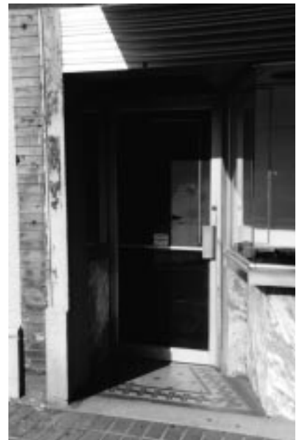
Inappropriate aluminum-framed door.
