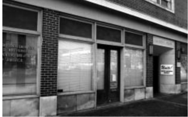
This storefront still retains its original double doors and its display windows and transoms.
