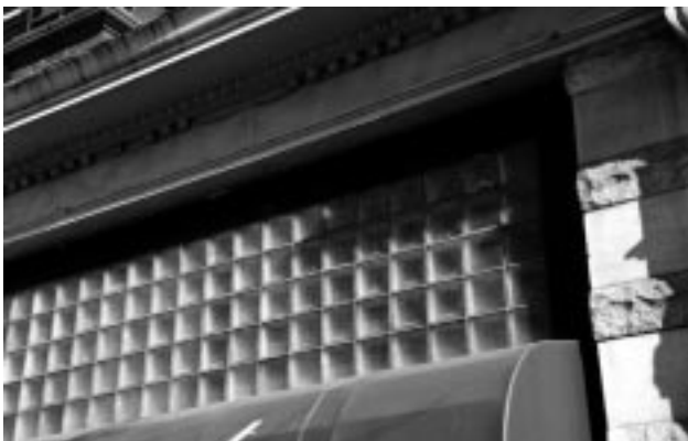
Glass block transoms are typical features of commercial buildings constructed during the 1920s.
