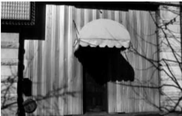
This original storefront has been inappropriately infilled with metal siding and a solid wood door.
