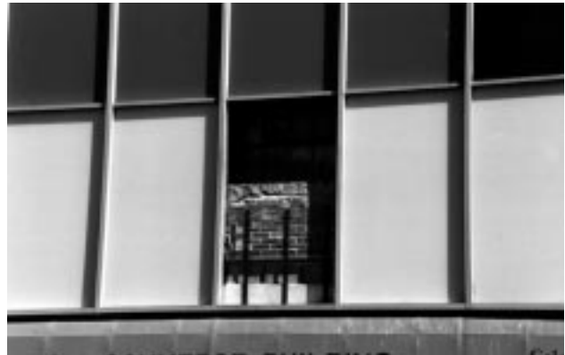
A close-up view to the gaps in the nonhistoric façade show that the original brick storefront is still intact.
