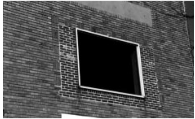
The removal of the original window and replacement with a smaller, fixed window has damaged the architectural integrity of this building.
