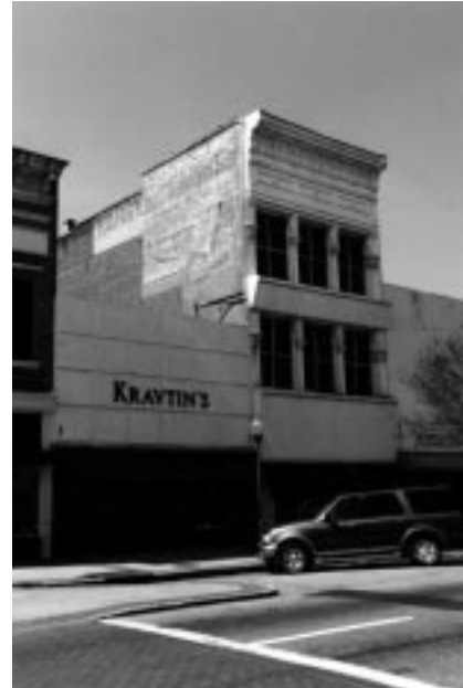
This nonhistoric façade conceals an original commercial façade that could enhance the appearance of the downtown as well as attract business to the individual retailers.
