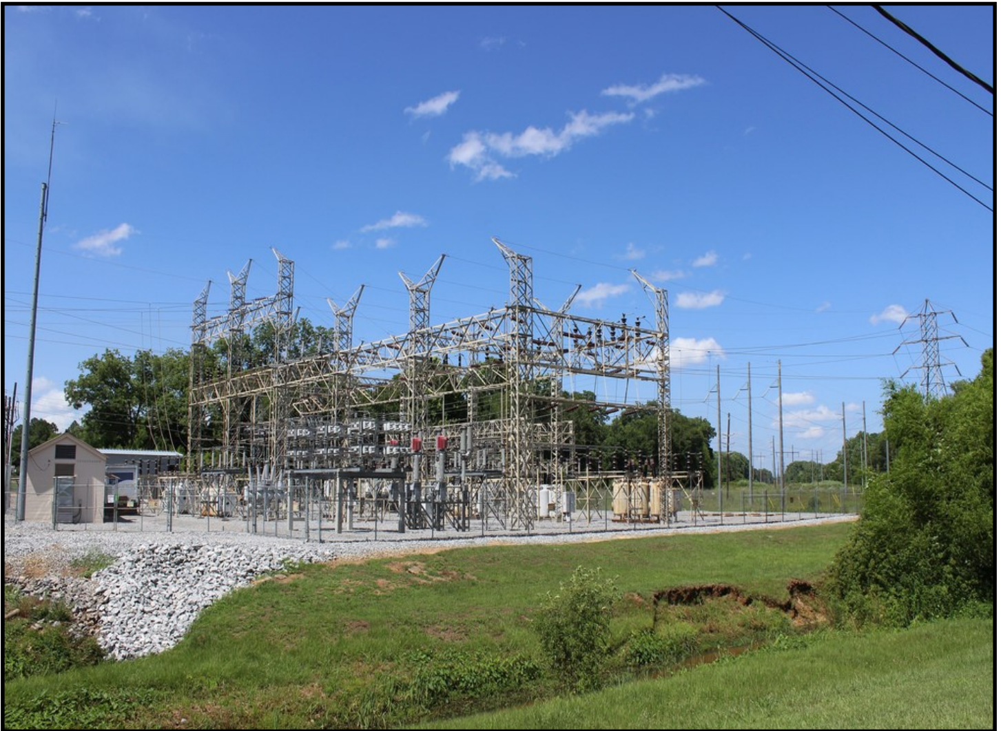
Georgia Power Substation
