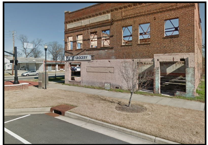
Dilapidated building along 6th Avenue
