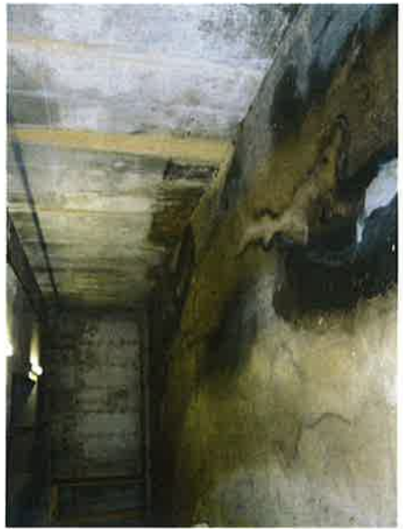
North wall of the parking deck showing water infiltration
